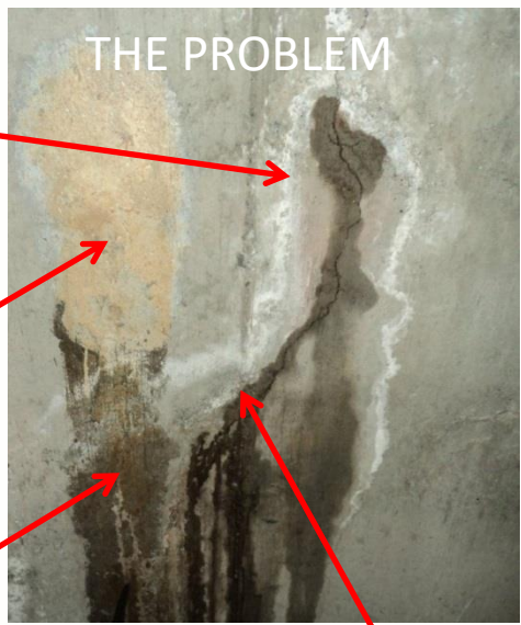
Freeze/thaw leading to cracks
